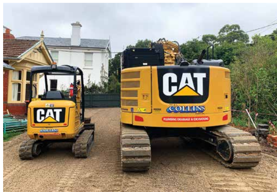
Fast forward ten years, and pictured are two of Collins' most recent purchases going to work recently on a house site in Kew.
