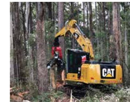
A new Cat 538FM fitted with a Satco processing head was delivered in March to MJ Contracting Pty Ltd, and is pictured operating near Wynyard in north western Tasmania.
