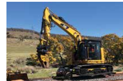
VEC CIVIL ENGINEERING PTY LTD new Cat RMT15F replacing the railway track, sleepers and ballast near Avoca in Tasmania's Fingal Valley.
