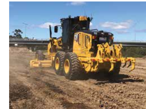
Geelong based Norris Plant Hire were quick to try out the new looking Cat 140 Motor Grader adorned with the new trade dress and livery. This machine joins two existing 140M Series graders in the fleet at Norris Plant Hire.
