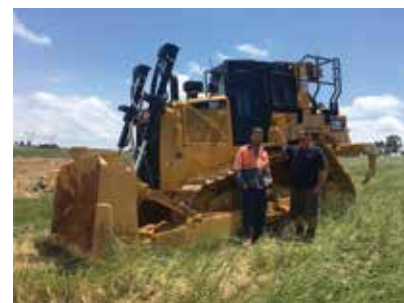
Gary Morrison, owner of Tooradin Excavations, puts his new 3D equipped D6TXL to work on a dam job in South Gippsland.
