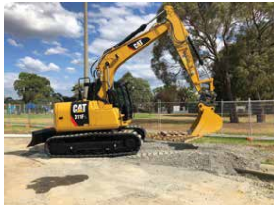
Ace Earthmoving Pty Ltd based in Morwell have updated an old Cat 311C with a new Cat 311FL RR, pictured here building a new roundabout in Traralgon.
